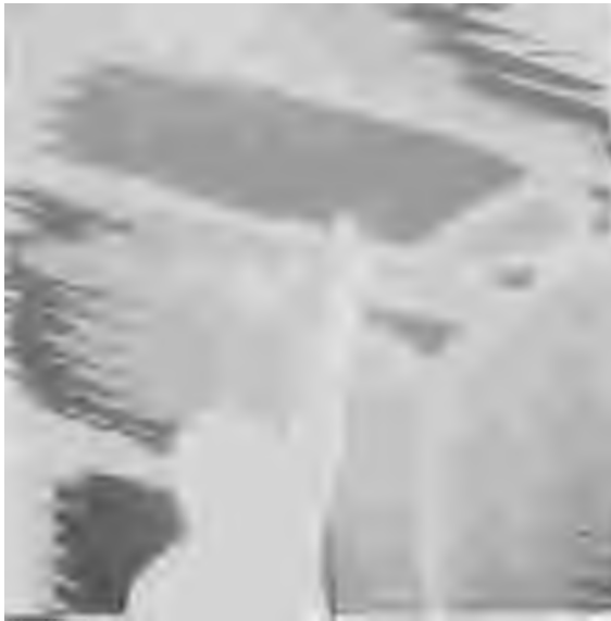
Figure 1-5B. Infrared Thermograph Reveals Anomalous Cold Patch in Upstairs Ceiling.
