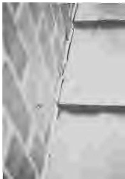
C: View from Outdoors. Caulking Comes Away at Wood-Masonry Joint.
