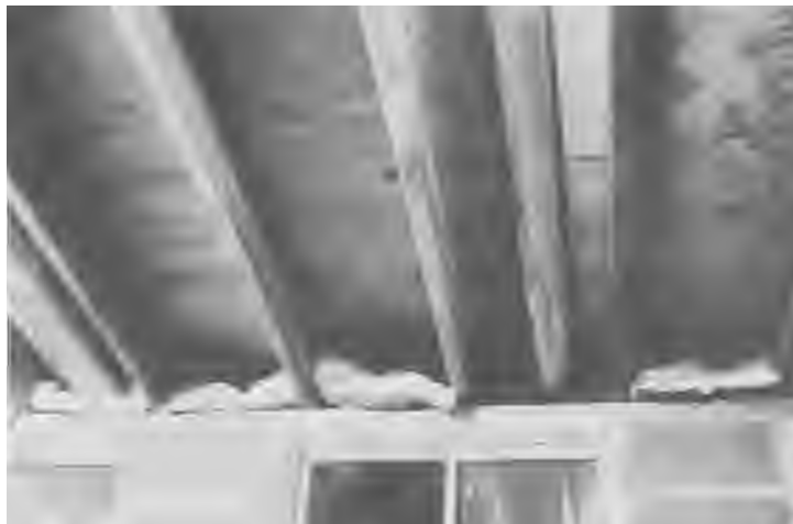
Figure 1-6B. Ducts Passing into Living Room Overhang, Casually Insulated.
