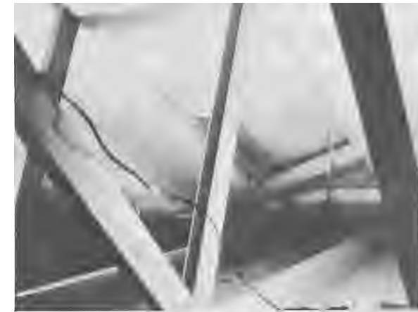
Figure 1-5C. Cause of Patch in Figure 1-5B is Traced to Missing Batt of Attic Insulation.
