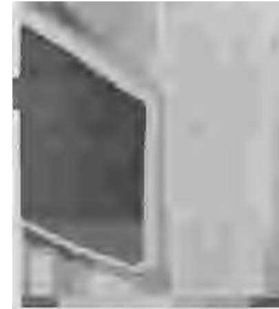
Figure 1-9C. Characteristic Corner Pattern: Cold Air Flows from Outside Through Space Between Firewall Masonry and Sheet Rock Panels and Merges with Warm Air from Basement.
