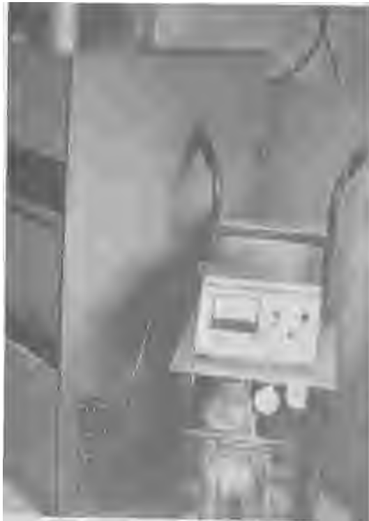
A: Air Infiltration Measurement Device, Alongside Gas Furnace.
