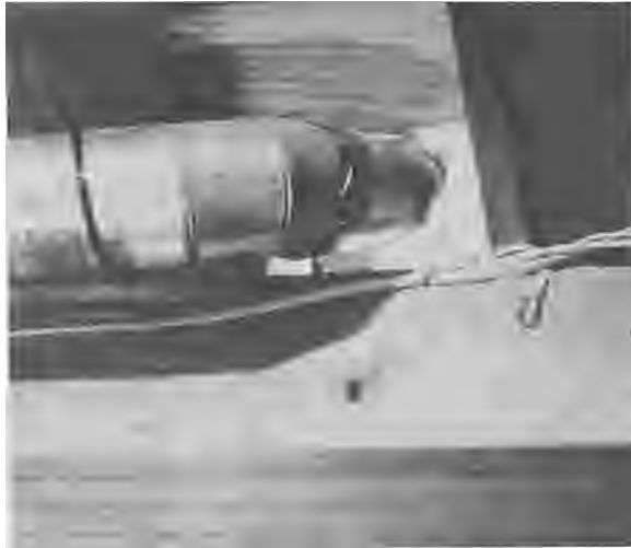
Figure 1-7A. View of Open Shaft Around Furnace Flue from Basement to Attic. In Foreground, Duct to Upstairs Bedroom Passing Through First Part of Shaft; Attic End of Shaft (Not Visible) will be Sealed as Part of Princeton Retrofit Package D.
