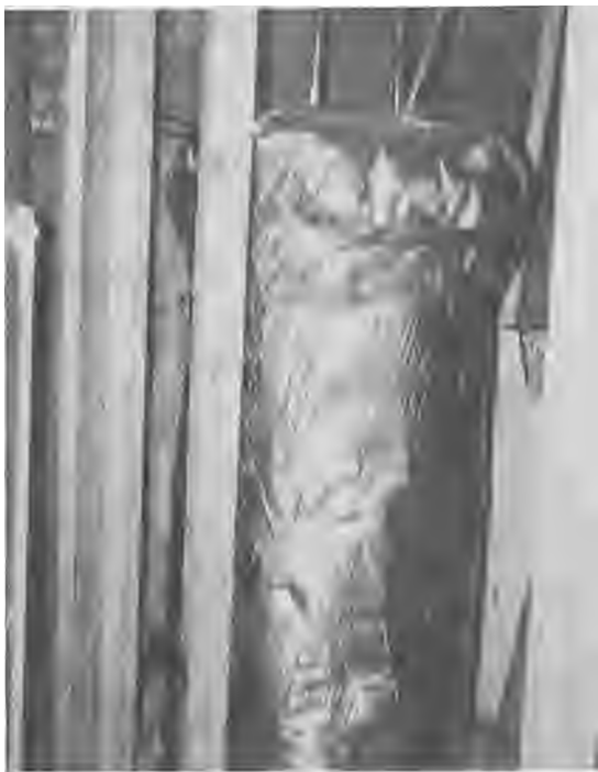
Figure 1-4B. Electric Water Heater Following Retrofit, Wrapped in Foil-Backed R-7 Insulation.
